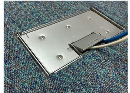
Trench-type floor box installed on Cable Trench
