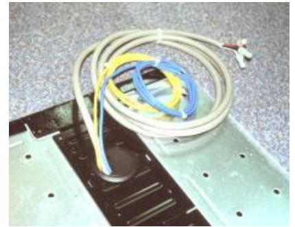
Cables extending through Exit-Cap to workstations or partition
